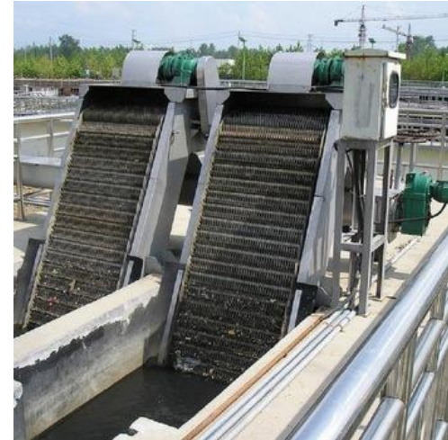
Figure 3: Example of Bar Screens in WWTP [3]
